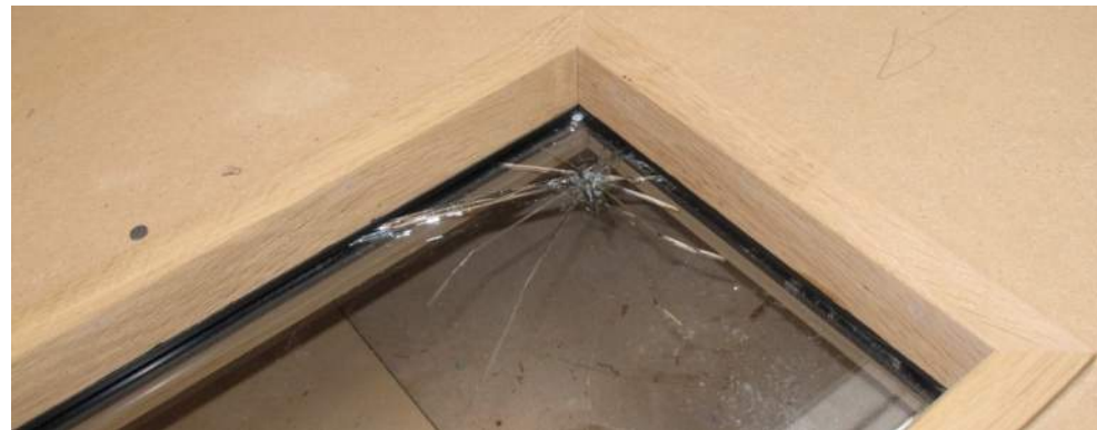
Example of broken glass
