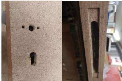
Void within leaf edge & frame following the removal of a lockset.
